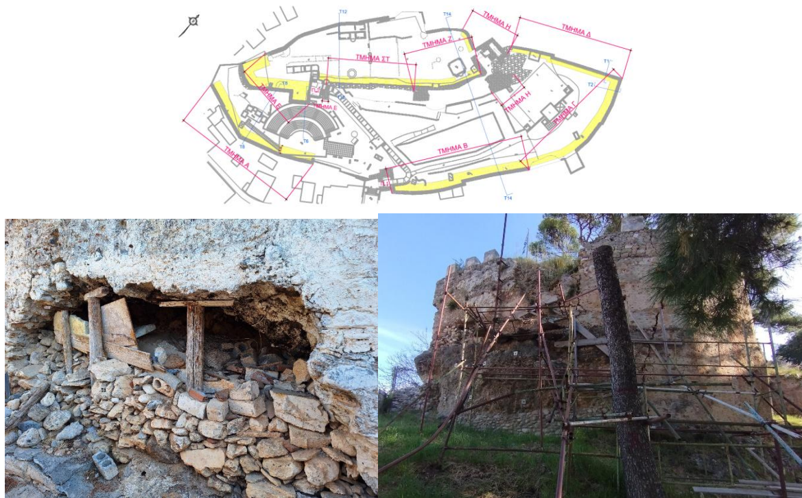
Figure 5. Discretization of the Castle into parts. Partial collapse in part A and cracking in part E.
