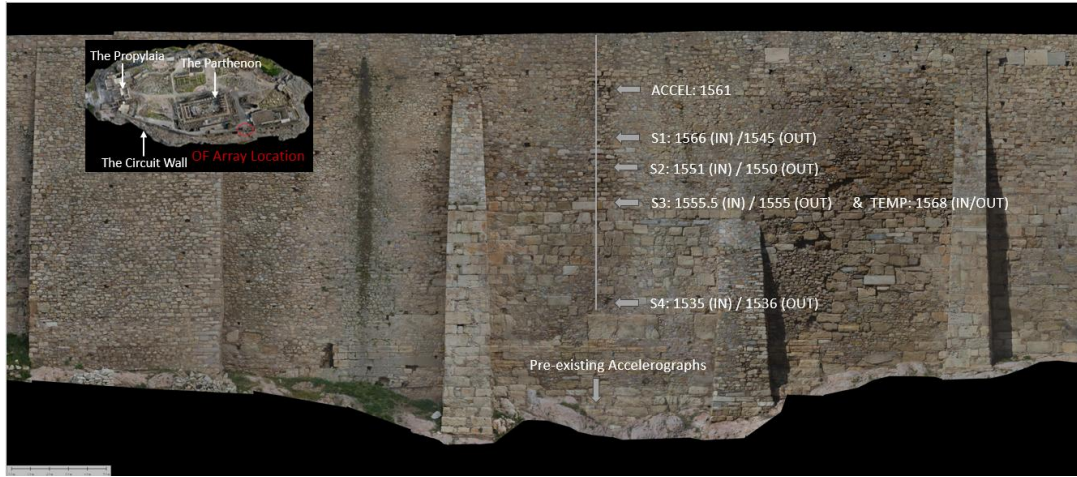
Figure 2. Positions of the sensors installed on the Circuit Wall, illustrating the overall monitoring layout.
