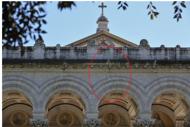
Figure 2: Crack opened in the pediment of the Quadriportico following the 2016, October 30 th event
