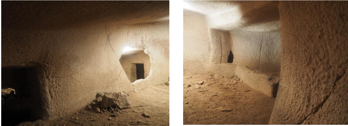
Figure 4. Observed damage of Tomb I, “Iloi Ispiluncas”, Sedilo (OR): passing crack (left) crack pattern (right).
