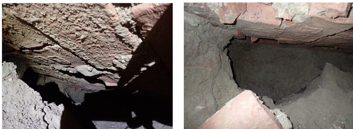
Figure 3. Trial excavation S13 highlighting a large void beneath the masonry building foundation
