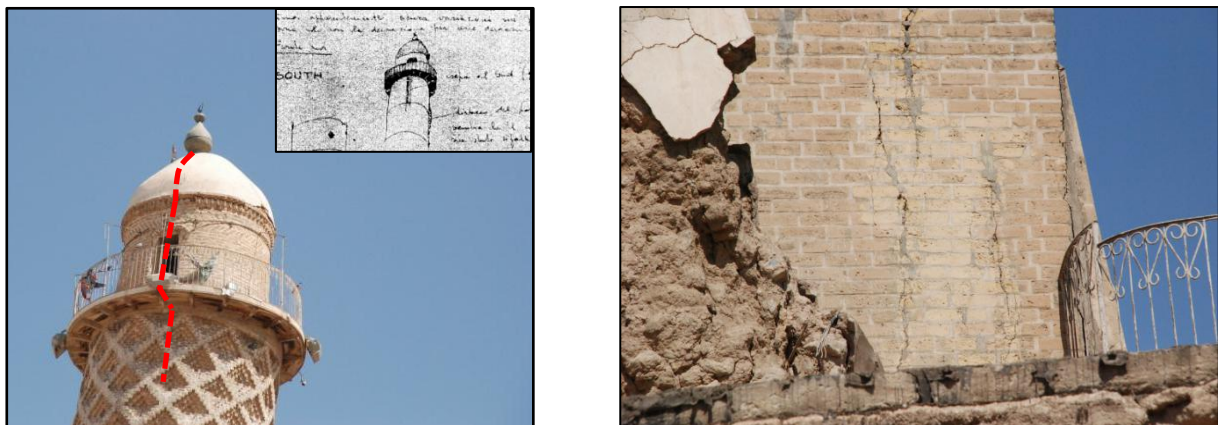
Figure 4. Tilting of the wall and crushed masonry (left). The outer brick texture hides a more chaotic masonry layout in the volume underneath (right).
