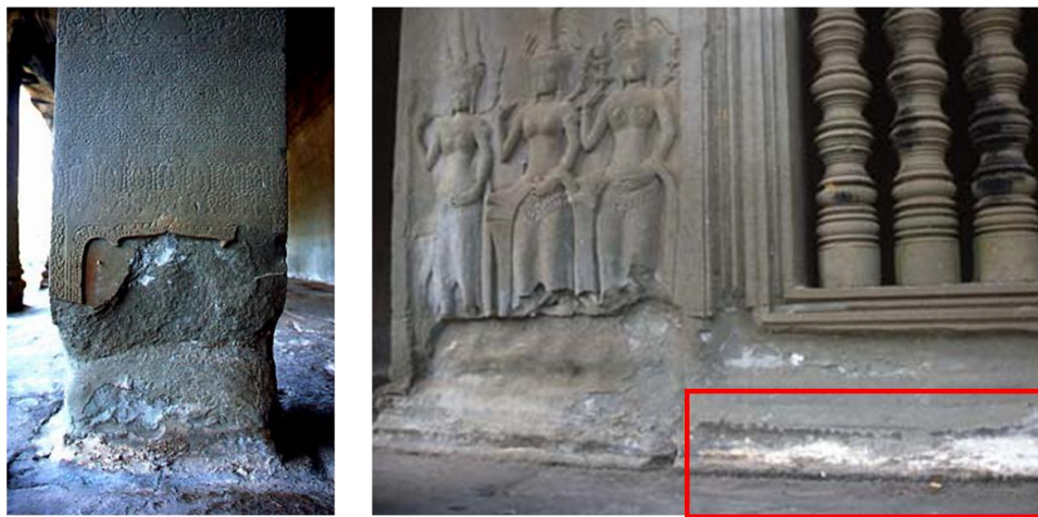
Figure 5. Damage to a pillar (left). Example of scaling on the carvings and salt efflorescence, in boxed area (right). (From Siedel et al., 2008)
