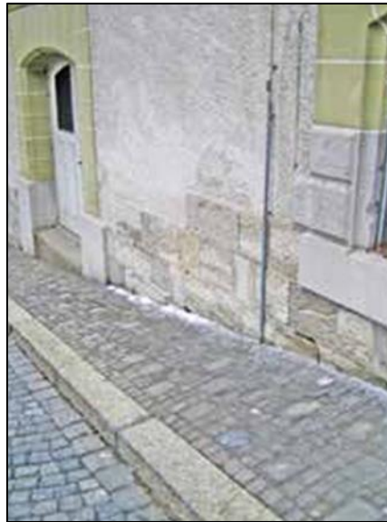
Figure 4. Accumulated salts at the base of the structure (From Charola et al., 2017)
