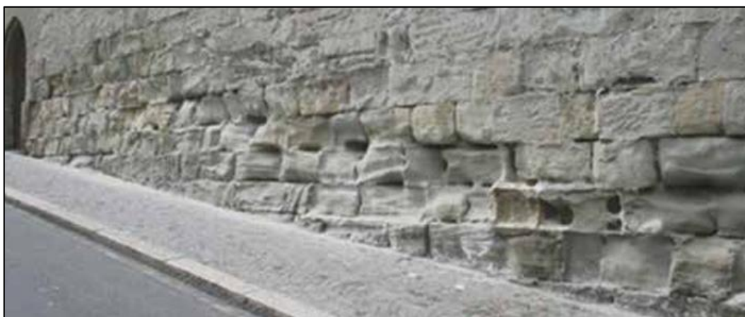
Figure 3. Salt weathering in upper portion of structure (From Charola et al., 2017)
