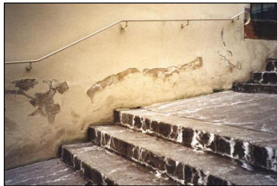
Figure 2. Accumulated efflorescence from dried deicing salts (From Steiger et al., 2010)
