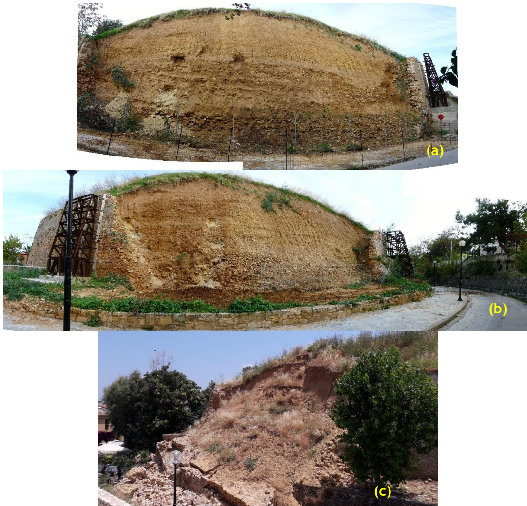
Figure 4. View from the level of Dounopapa st in November 2017 a) of the eastern failure and b) of the western failure after removal of soil and wall debris and construction of the steel buttresses, and c) view of the northern failure in March 2019 before the removal of the debris. Small excavations on the slopes in Fig. 4a and 4b mark the locations of samples taken using an excavator from the various layers of the cavaliere materials.
