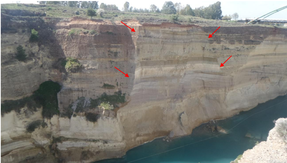
Figure 1. View of the slope failure, which occurred on February 26 2018 at the south slope of the Corinth Canal.
